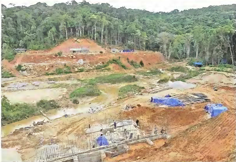
Plate 3. Hydro-electric dam construction in the Da Nhim Watershed Protection Forest. A male Grey-crowned Crocias could be heard singing from a tree top behind the photographer. (Jonathan C. Eames)
